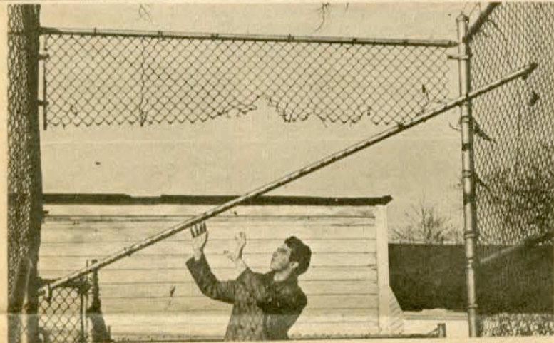
THIS FALLEN FENCE post poses a hazard for anyone who walks under it, as 12A Dean Kowalszyk demonstrates. The post has been there for six weeks.
